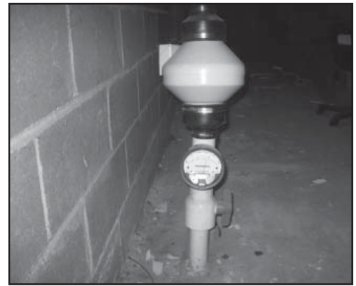
Figure 2. Typical Sub-Slab Depressurization Fan and Vacuum Gauge, Case History Number 1.
